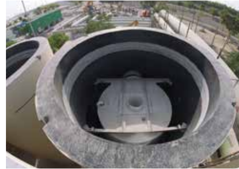
Shaft Pumping Station - Qatar
