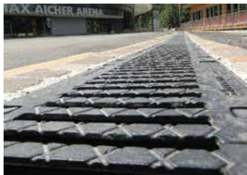
Linear Drainage & Slot Drains
